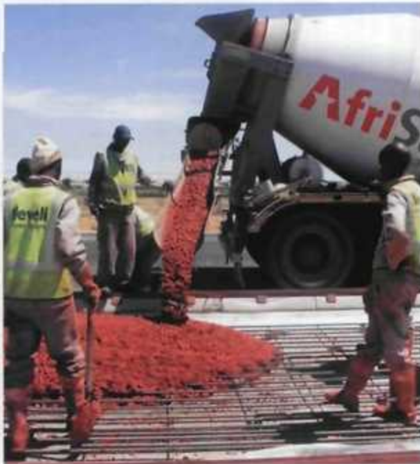
Quality control is an important aspect of the contract awarded to AfriSam for the readymix concrete for the BRT.
