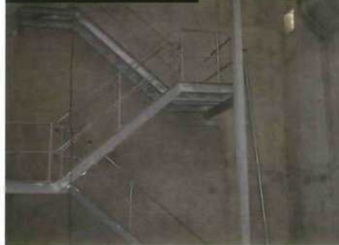
Steps to machine hall at Sol Plaatje
